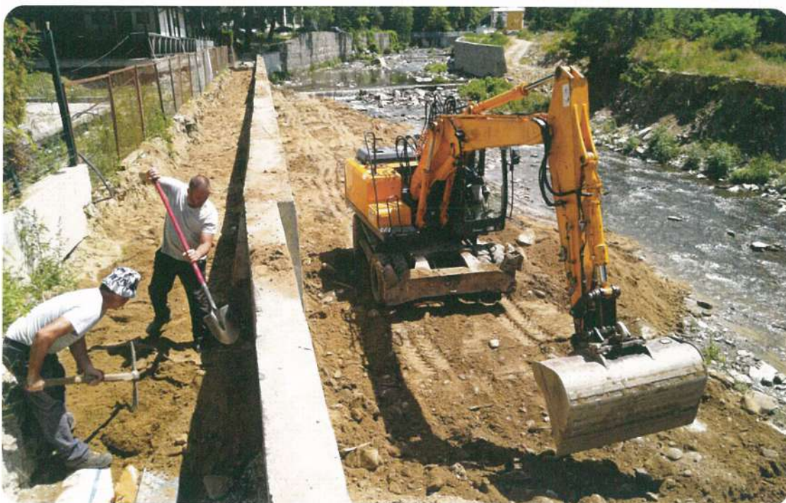
Major repair of a heating pipeline for mineral water from a water source falling within the land property parcel with identifier 38844.101.95 under the cadastral map of the town of Kostandovo, Rakitovo municipality, Pazardzhik region
