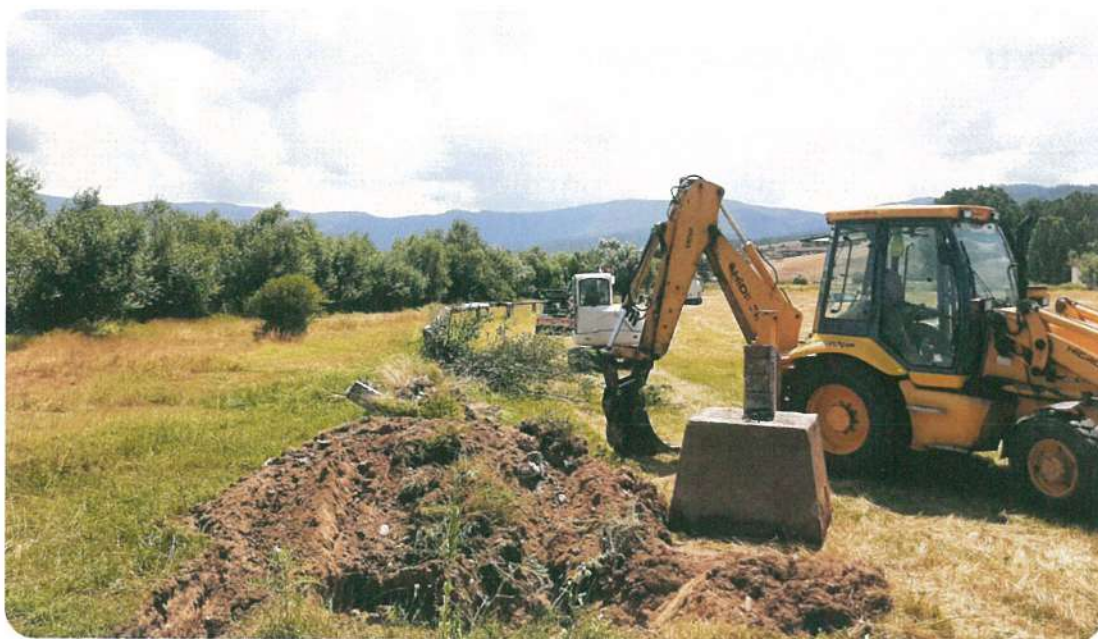
Street water supply pipeline for mineral water with a length of L 1300, village of Ognyanovo, municipality of Garmen
